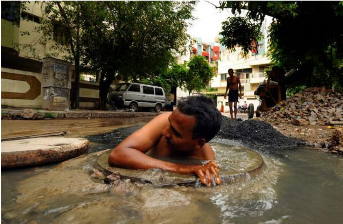
In this July 7, 2010 photo, a sewerage worker clears a choked drain at Anandnagar, Hyderabad. Photo: Mohammed Yousuf
